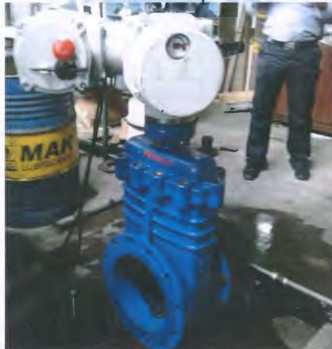
VALVE UNDER TEST
